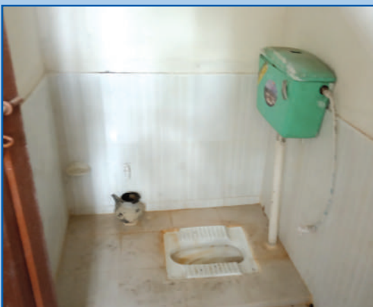
Inaccessible door-width and sitting arrangement of space inside a toilet in a health centre of Sitakund Upazila © HI
