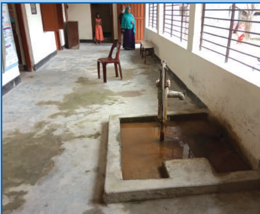
No tactile marking in a health centre of Sitakund Upazila © HI
