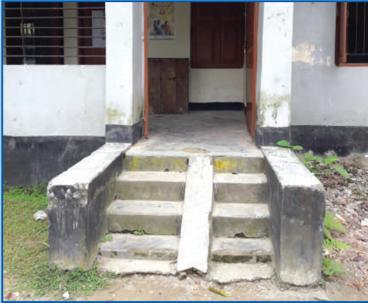
Main entrance of a facility compound in the Sitakund Upazila, as not user friendly for wheelchairs, crutch users and white cane users © HI
